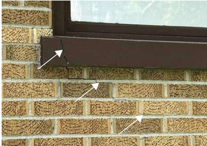
Cracked sill and step cracking of brick - typical at all windows
