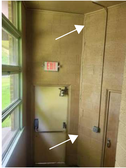
Interior cracking at NW door
