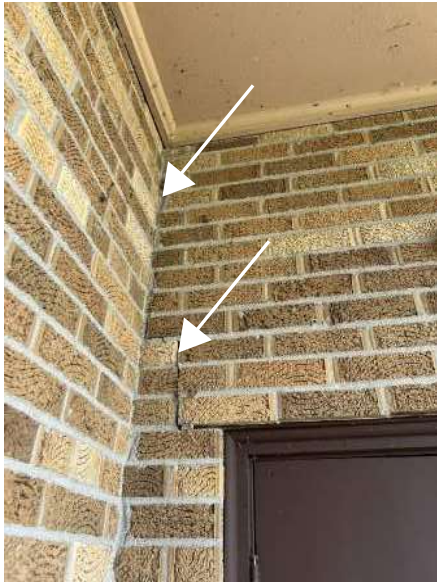
Exterior cracking at NW door
