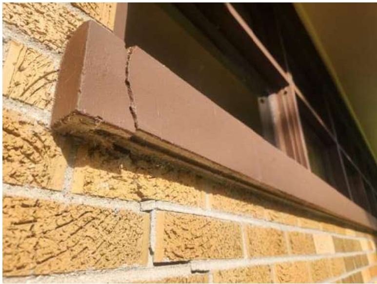
Detail of cracking sill condition
