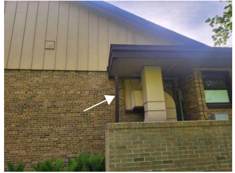
Warped 4x4 post at rear mechanical area
