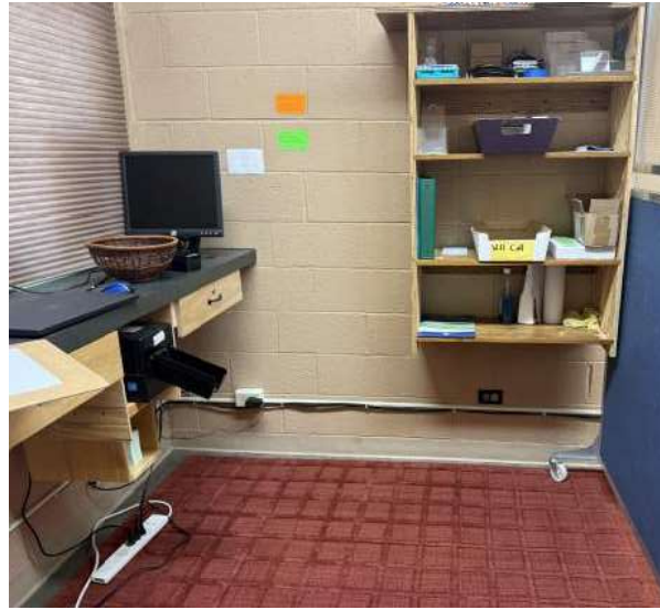
Widely used extension cords and plug strips within the ticket office
