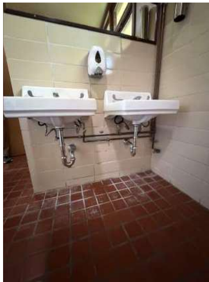
Wall mounted restroom sinks
