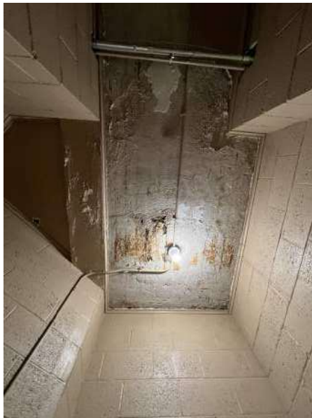
Water damage at backstage ceiling
