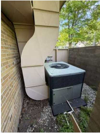
Exterior mechanical equipment
