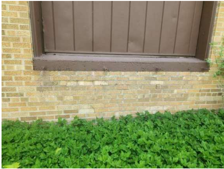
Stage door sill and brick deterioration
