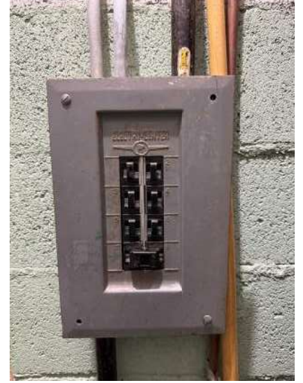
Old electrical panel
