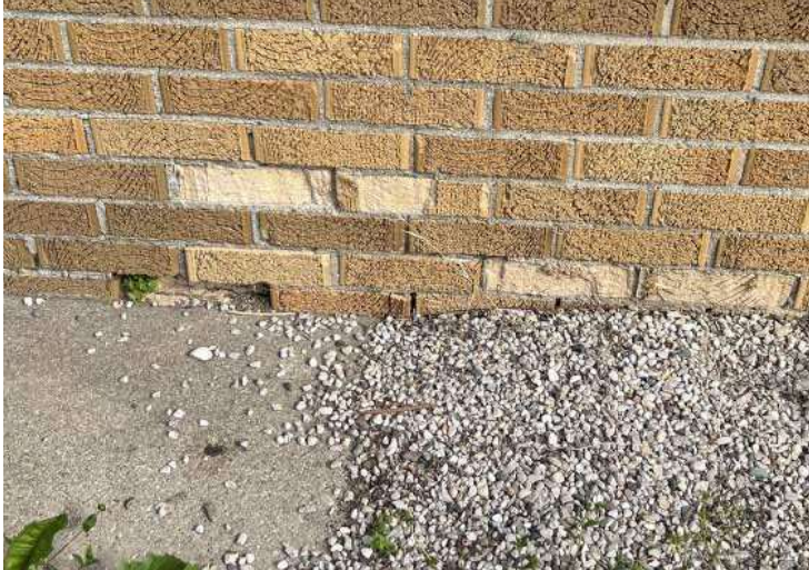
Minor brick deterioration at wall base, south elevation
