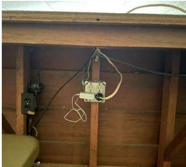
Widely used extension cords and plug strips within the spotlight booth
